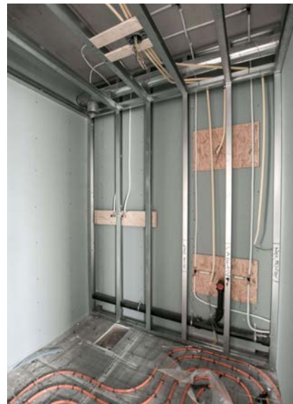
installations separated from structure
